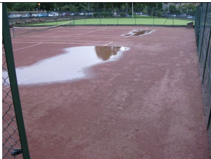
The 100 year old blaes no longer drains properly and ponds after heavy rain - sometimes for days.
